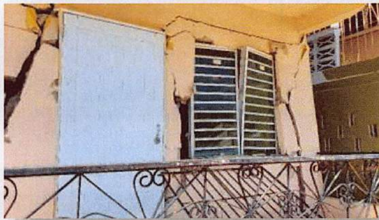
The earthquake caused doors and windows to fall apart and were therefore blocked or out of their frames
