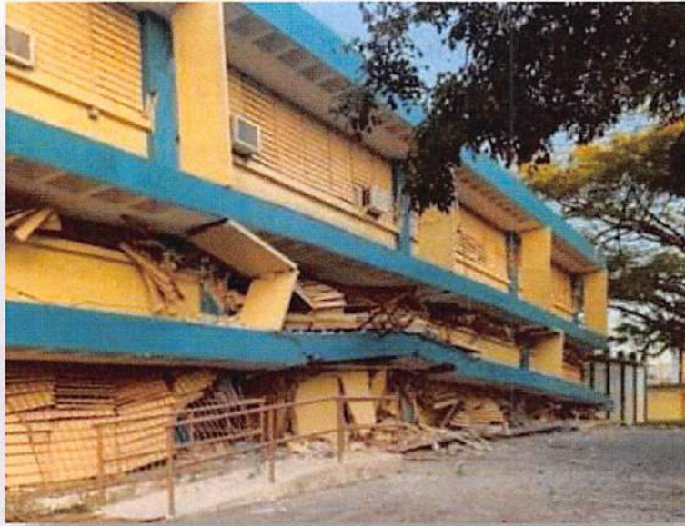
Agripina Seda School in Guánica collapsed on its foundations
