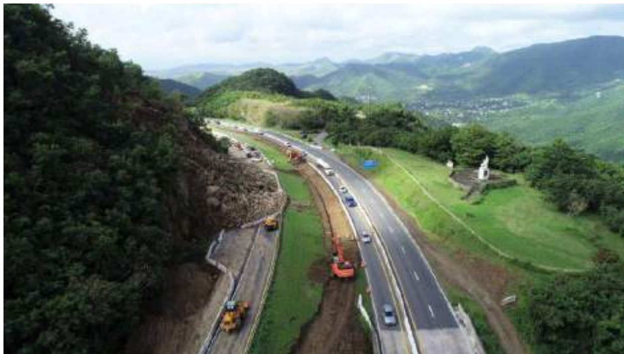
Figure 193: Landslide Between Salinas and Cayey, November 5, 2022 665
