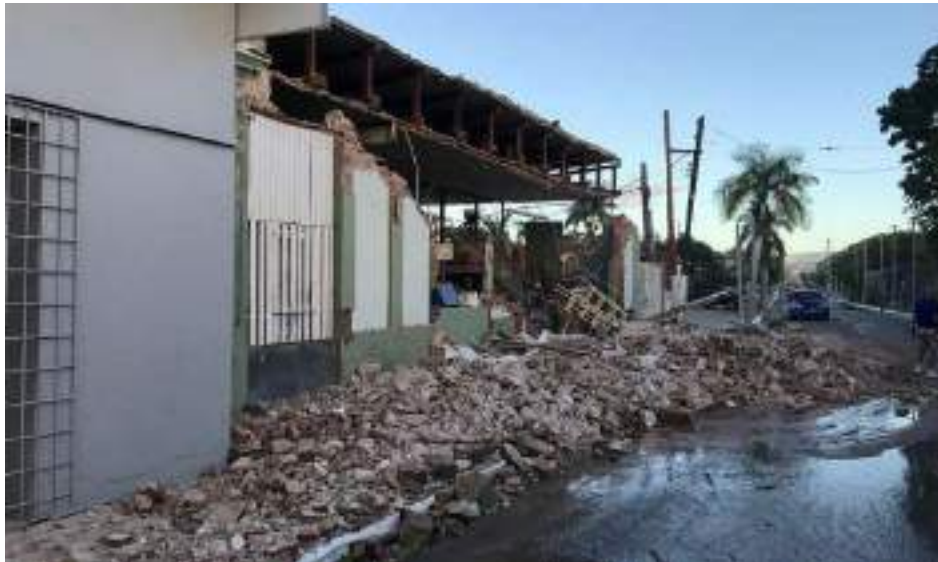
Figure 249: Shop in Guánica, Puerto Rico, Damaged by an Earthquake 897
