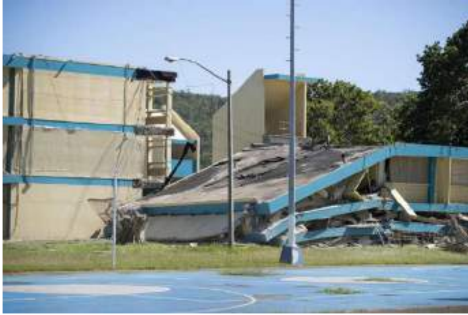
Figure 119: Earthquake-Damaged Middle School in Guánica, Puerto Rico, January 21, 2020
