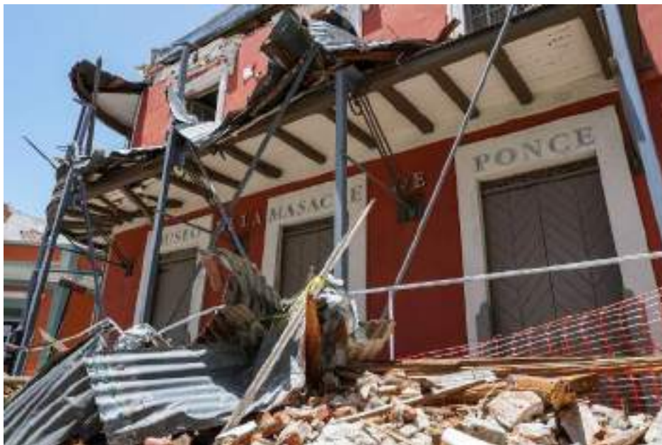
Figure 102: Earthquake Damage to Ponce's Massacre Museum 288
