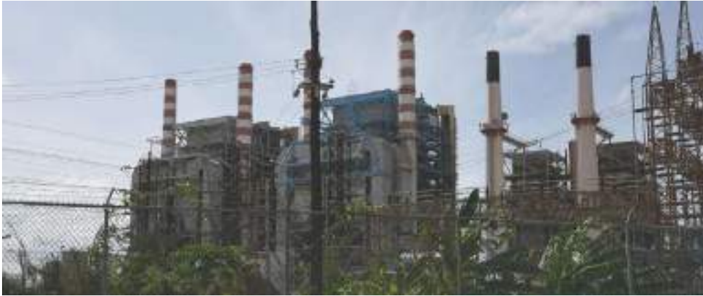
Figure 111: Damage to Costa Sur Power Plant from January 2020 Earthquake 299
