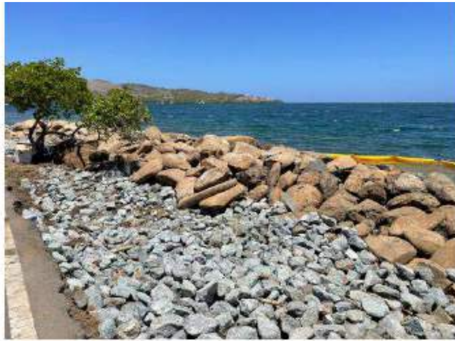
Figure 84: Relocated Revetment Above Mean High Tide in Culebra
